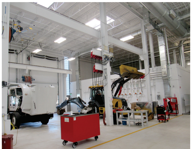
Design strategies throughout Denver Water's Operations Complex were selected to improve work efficiency and well-being. As an example, the Fleet Building includes standardized tool carts, centralized fluids, natural light and white concrete that reflects light up and under vehicles. Photo credit: Denver Water
