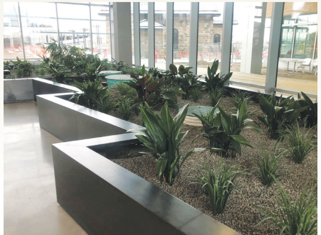
Wetland planter beds in Denver Water's Administration Building lobby provide additional filtration and nutrient removal for the building's onsite wastewater recycling process (WEc1, WEc2).
