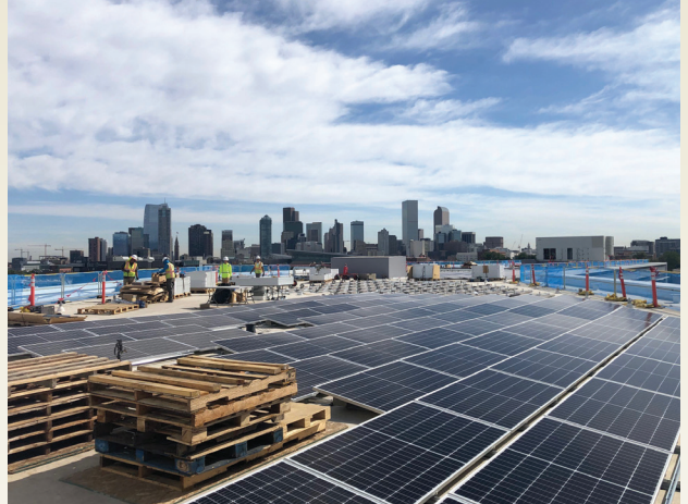
Solar panels were installed on Denver Water's Administration Building to achieve a net zero energy goal for the building. Photo Credit: Denver Water (EAc1, EAc2).
