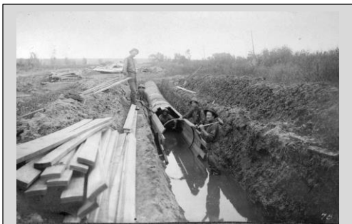
Workers build a wood-stave pipe in this undated photo. In the early 1900s, many of Denver Water's conduits and large pipes were made of wood.
