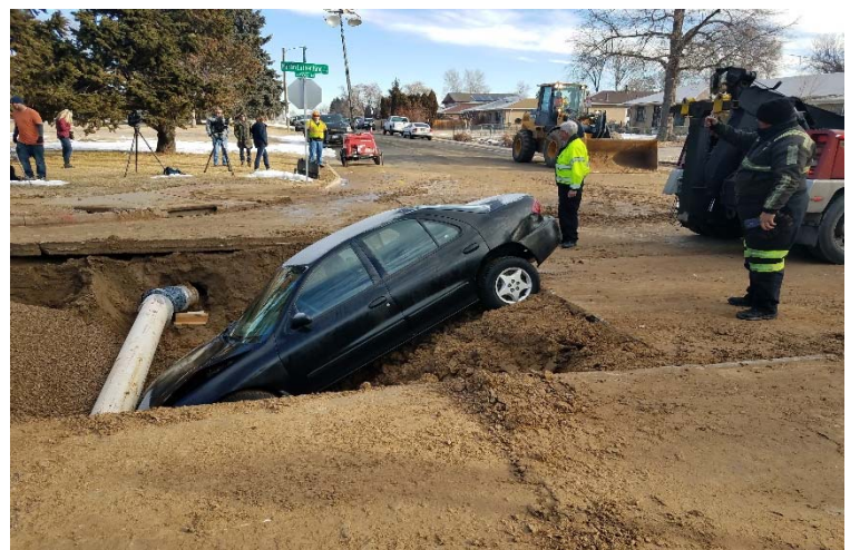
During two different Denver Water service line repairs, vehicles went around Denver Water barricades.
