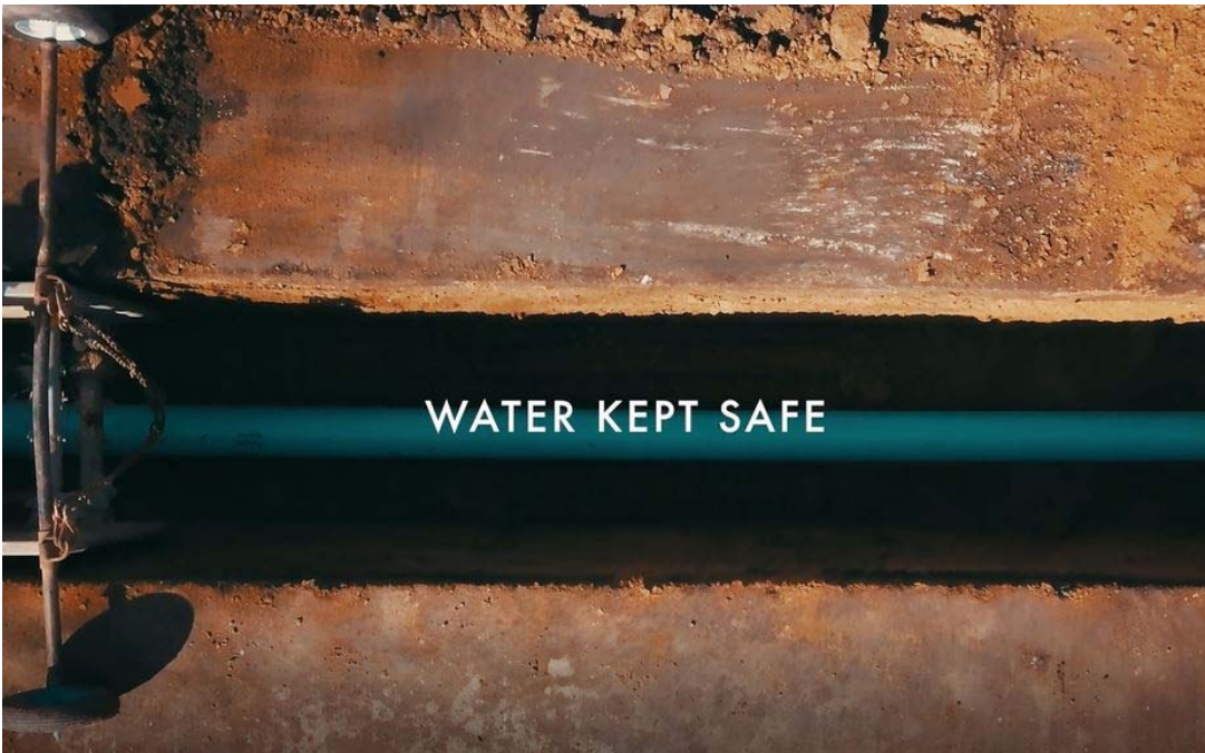
Figure shows an aerial view of a Denver Water pipe being placed
