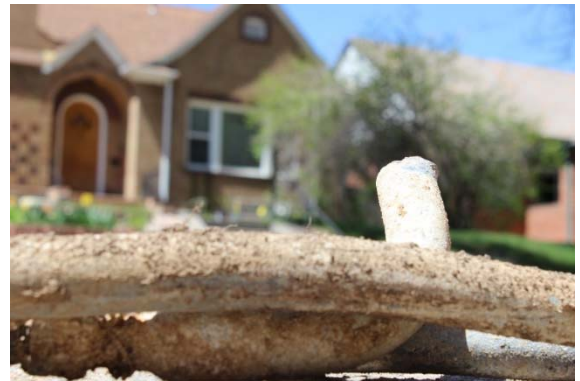
The water Denver Water provides is lead-free, but some homes are at risk of lead entering the water through their household plumbing or service line, like the one pictured here. The house in background was built pre-1951.
