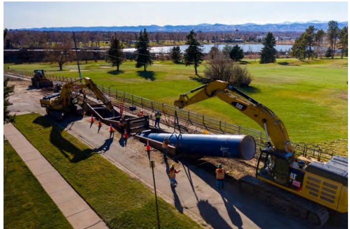
Construction crews install a 50-foot section of steel pipe next to Willis Case Golf Course in northwest Denver, 2020
