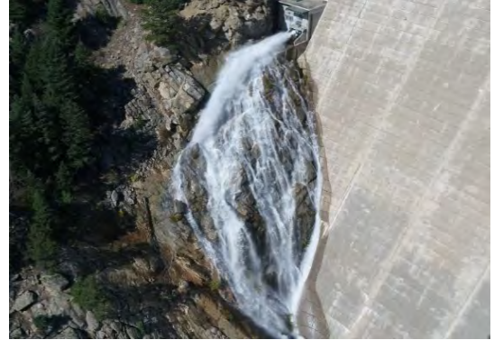
Gross Reservoir Expansion - Auxiliary Outlet Works taken by Project Engineer Jeff Martin
