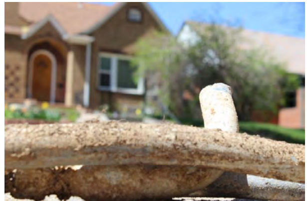
Lead service lines, like the one pictured here, are more likely to be found at homes in the Denver area built prior to 1951.
