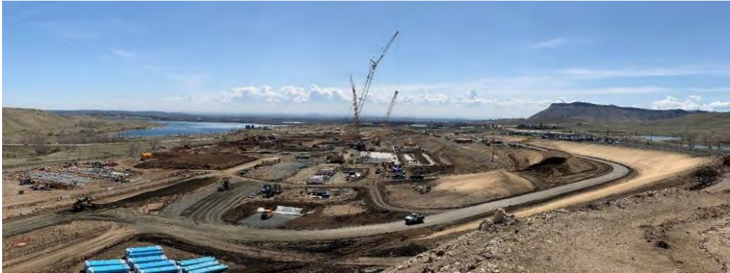
Panoramic view of Northwater Treatment Plant taken by Water Treatment Engineer Peter J. McCormack.
