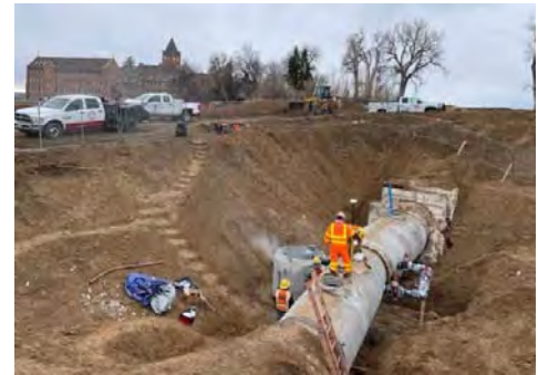
Denver Water Construction Project Inspector checks new pipes and valves for proper alignment, 2022.
