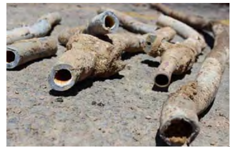
Lead service pipelines removed as part of Denver Water’s Lead Reduction Program, 2021.
