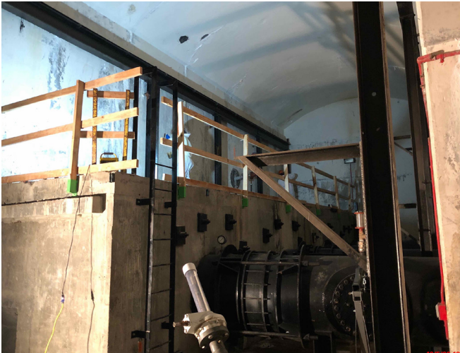
The original outlet works that was removed and replaced. Photo credit: Denver Water.
