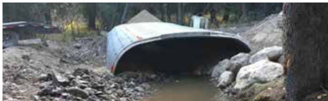
A nearly completed amphibian passage includes a more natural streambed along the bottom of the passage making movement easier for aquatic species. Photo credit: Denver Water.
